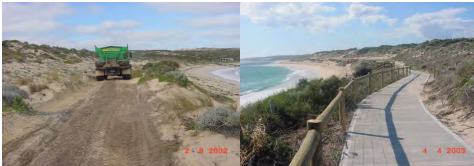
Figure 3.1 Coastal Walkway during construction in 2002 (L) and following installation of concrete path and fencing in 2003 (R).
